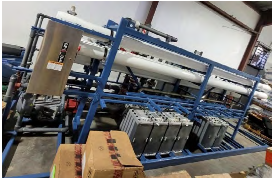
Reverse Osmosis Plant
